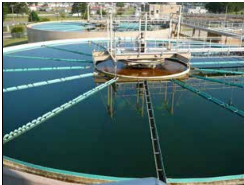
Figure 34: Circular drinking water clarifier with radial launderers and v-notch weir plates Photo by author.
