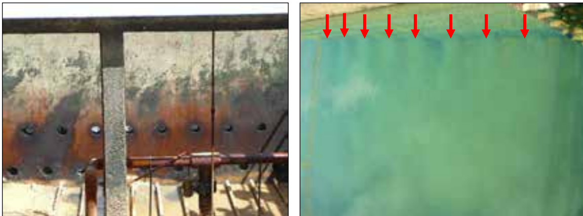
Figure 27: Clarifier w/ perforated inlet baffle wall The rectangular clarifier pictured has a perforated inlet baffle wall. The design is intended to uniformly distribute the flocculated water across the basin to provide uniform settling time and to minimize short circuiting. At left, the perforated inlet wall. Sludge collection pipes (white) visible at the bottom. At right one can see jet streams (red arrows) of the flocculated water entering the basin through the holes. This design would be credited with a baffling factor of 0.7 or better for purposes of calculation of CT. See discussion below under Clarifier Design Impacts Disinfection. Photos by author.
