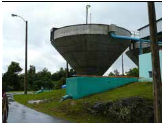
Figure 28: SpiraCone Solids Contact Clarifier Photo by author.
